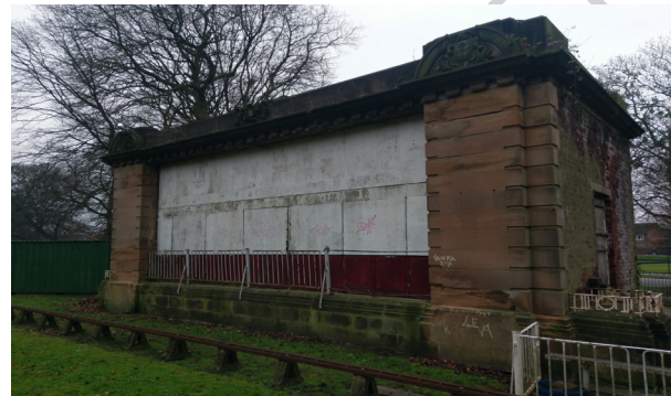
Fire-damaged open air theatre
